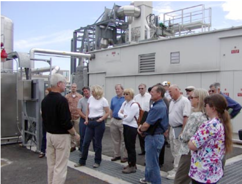
Greg Bush, King County, provides a close-up look of South Plant's new fuel cell.
