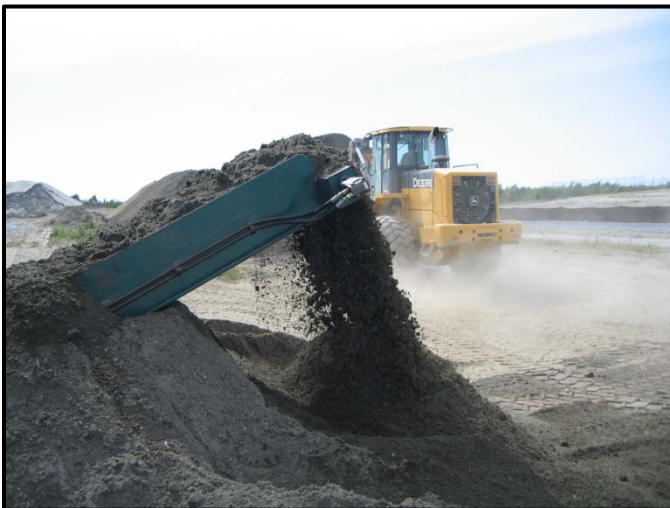
Figure 3: The soil mixer conveyor releases the newly fabricated soil into the stockpile area below.
